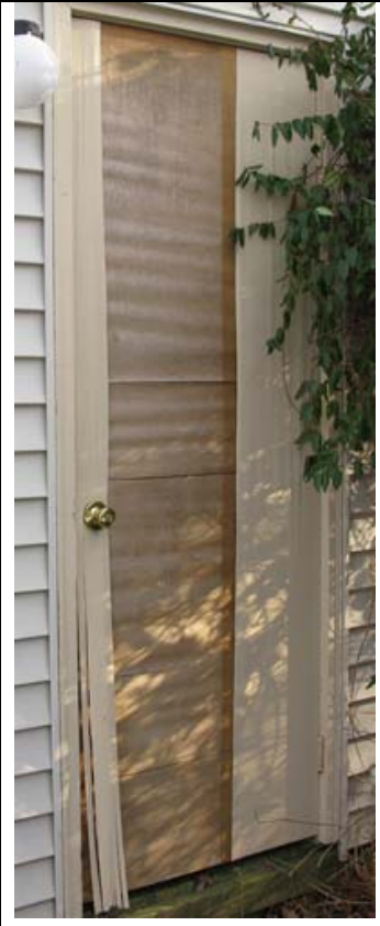
Interior grade doors used outside eventually delaminate and should not be used.
